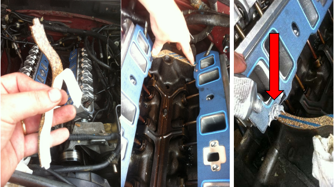
Photo 14: Applying cork gaskets and putting RTV silicone in corner of each. It is also perfectly acceptable to just use RTV by itself if desired.
